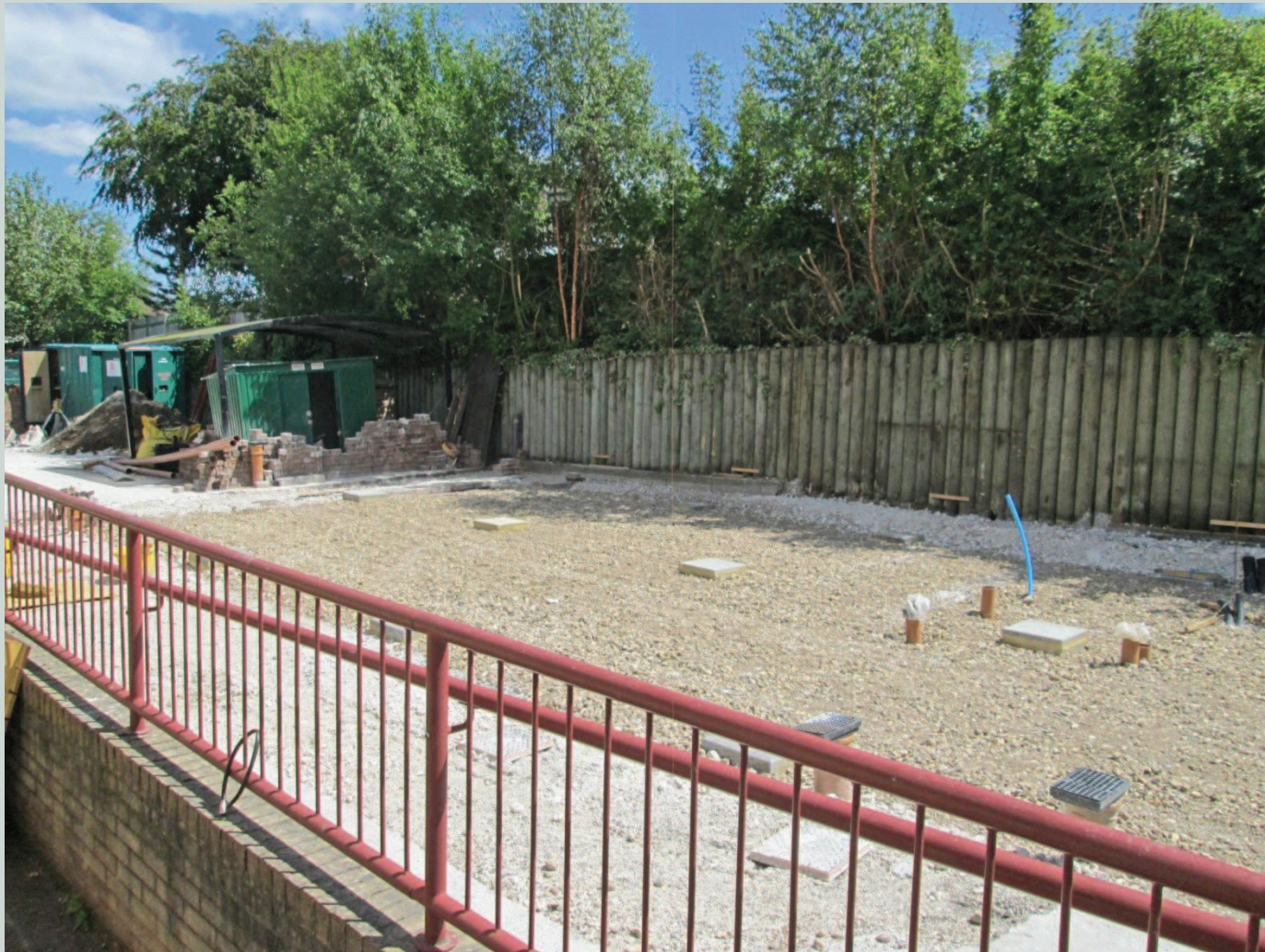
Fig 3 : Looking northeast toward location of the demountable unit, with footings in place
