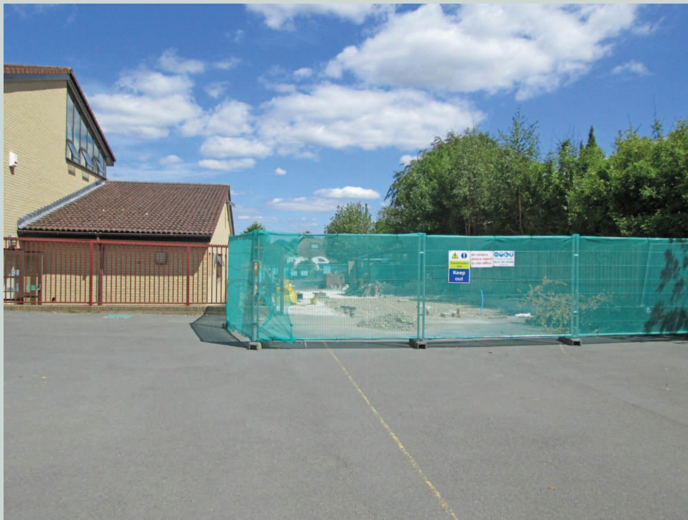
Fig 2 : View looking north from hard play area toward location of demountable unit
